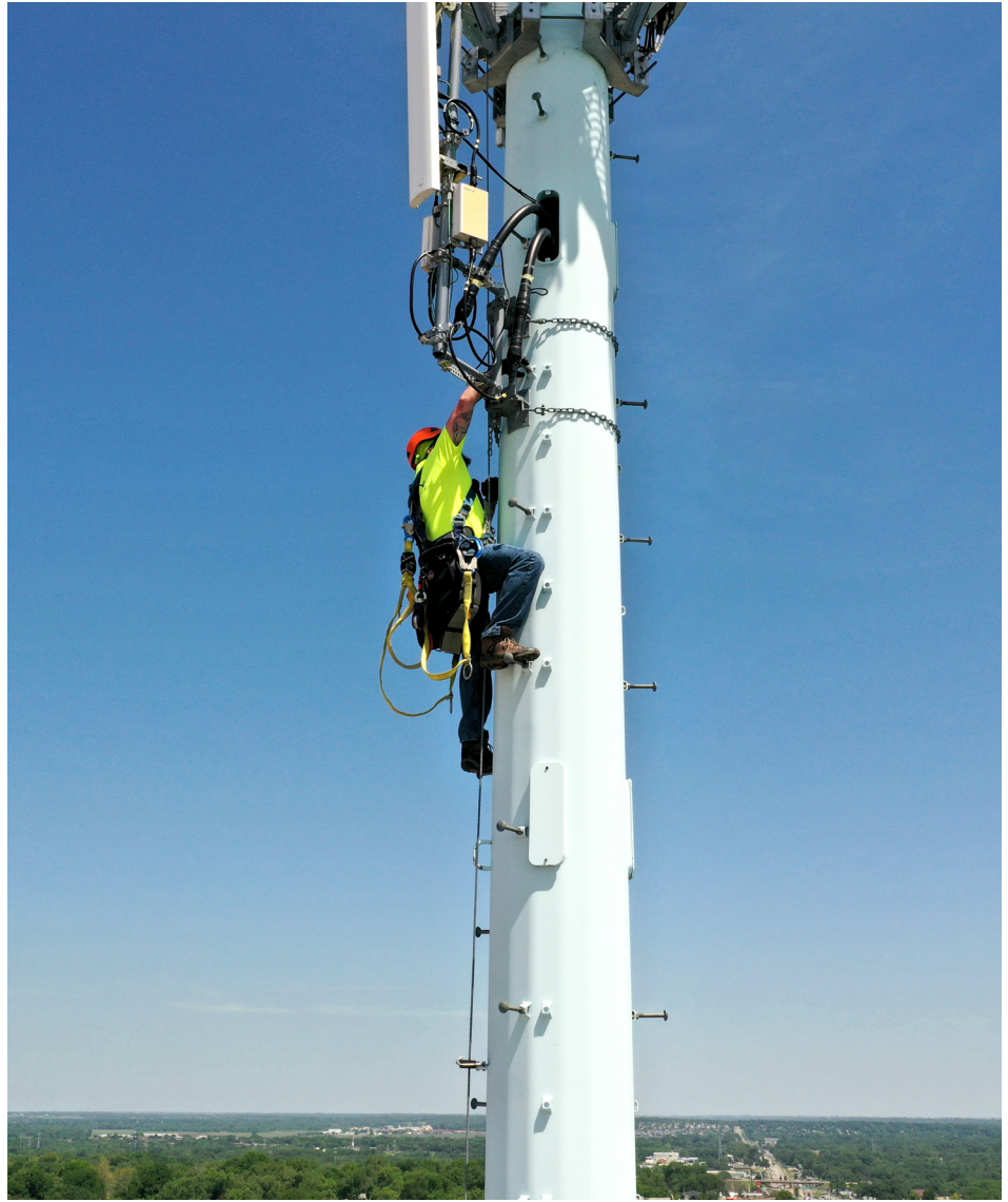
Murphy Tower Service is poised to be a big player in the state's digital future, whether helping expand broadband to rural areas or building out the Midwest's 5G footprint. CREDIT MURPHY TOWER/STUDIO IOWA
